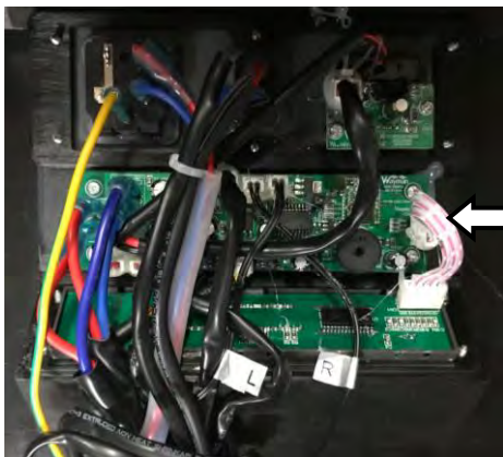
Main circuit board
